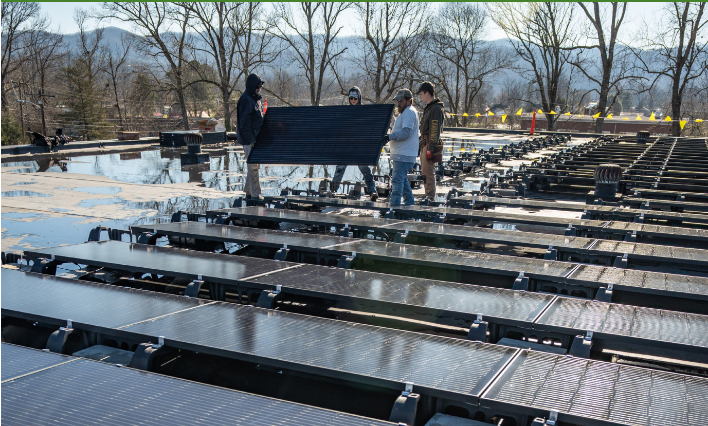
Solar Installation on Middlesboro Community Center © Mike Wilkinson
