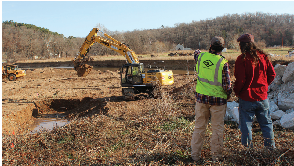
Construction began in December 2017 on the Elk River streambank stabilization project. © Kristy Stoyer/TNC
